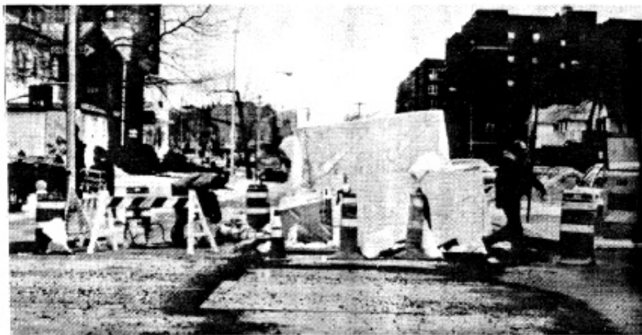
A makeshift wooden structure shelters NYNEX workmen as they labor to repair over 7,000 lines either damaged or destroyed by an underground explosion in Midwood last Wednesday night.
